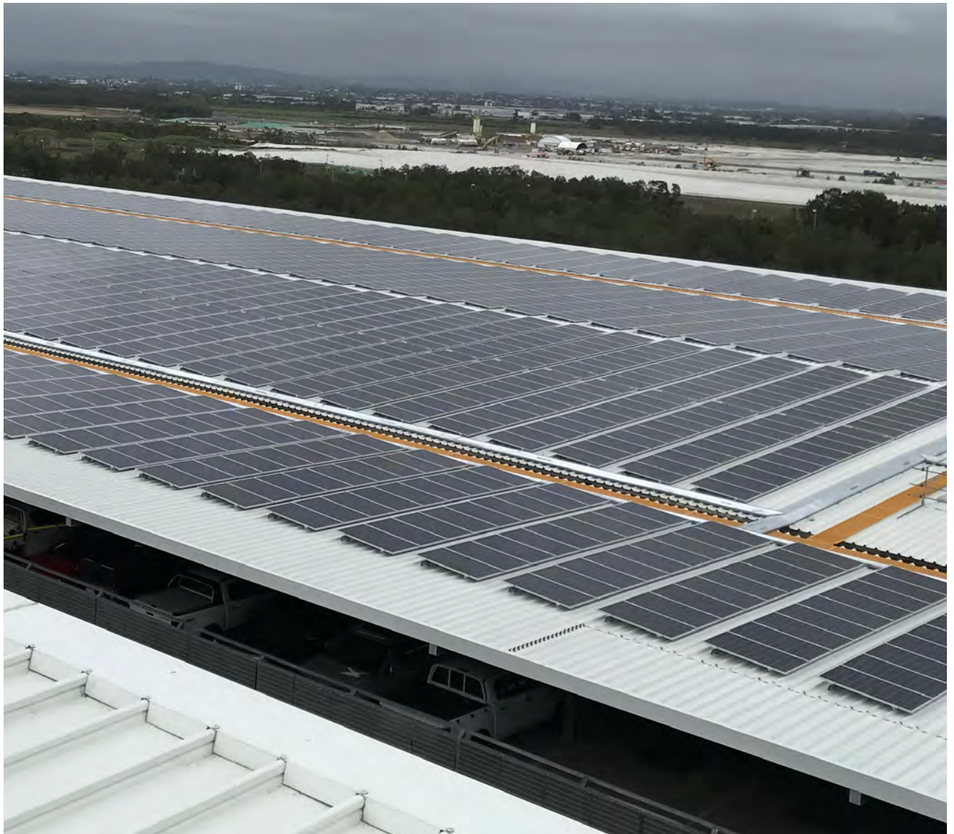
View of the Solar Panel Installation on the Domestic Terminal P2 Multi-Level Carpark Roof. Progress on the New Runway project can also be seen in the background.
