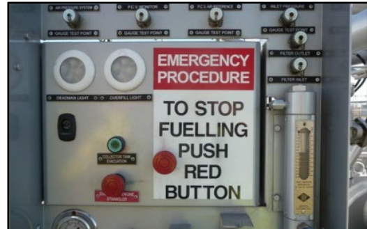
Figure 11 Emergency Stop on Vehicle
